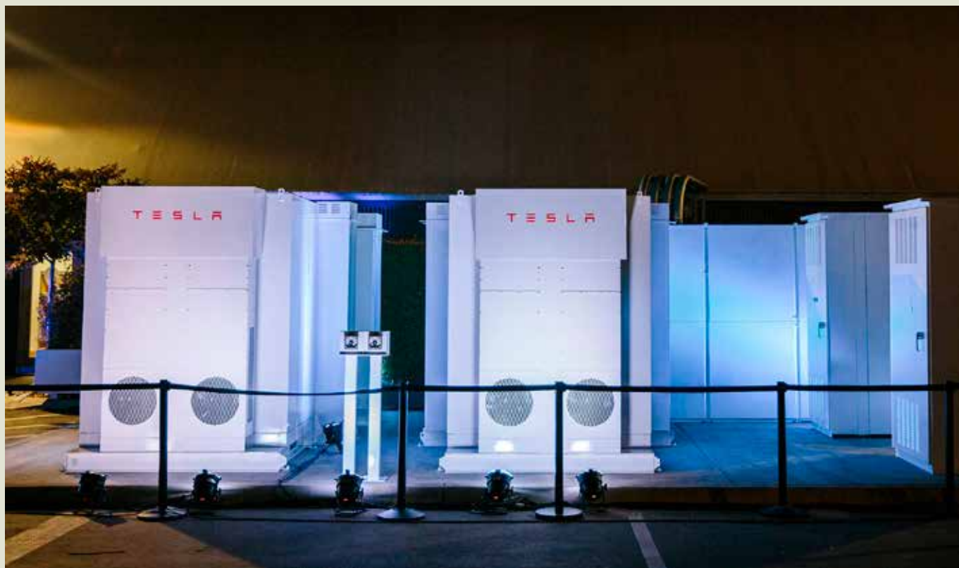
LOGAN CITY COUNCIL IN BRISBANE HAS COMBINED EMERGING SOLAR POWER AND TESLA BATTERY STORAGE TECHNOLOGY TO DELIVER A RELIABLE, SAFE SOLUTION FOR WATER DISINFECTION IN THE CITY’S FAST GROWING SOUTH WEST CORNER
